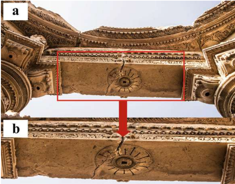
Fig. 21 Fracture at the Mahamandap of the Someshwar temple (Temple no. 2). a Fracture at the top part of the connecting slab of the pillars. b The fracture is deep and vulnerable
