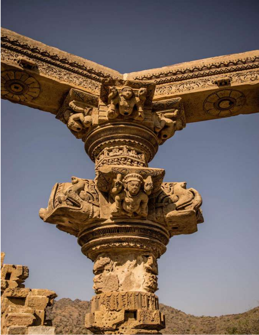
Rep. Fig. 6 Decorations (A warrior in the jaw of Makara) at the partially damaged pillars of the Mahamandap of the Vishnu temple (Temple no. 6)
