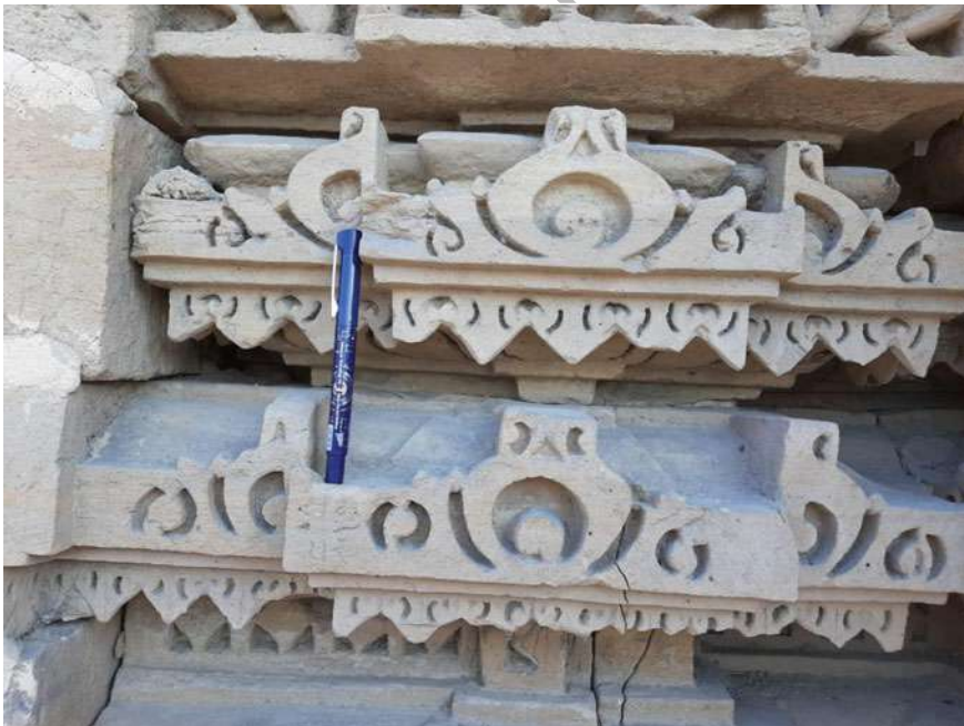
Fig. 8 Block to block locking system of rocks in the Shiva temple (Temple No. 1) (Pen of length 13 cm)
