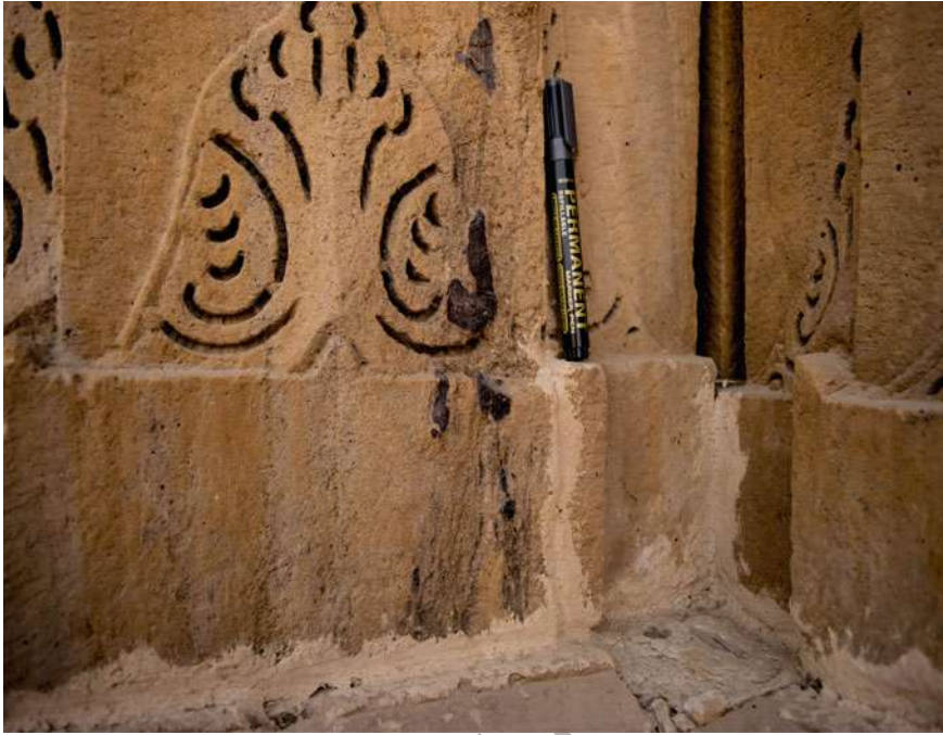
Fig. 15 Restoration of sandstone block (black pen marker) (Temple no. 1) with calcareous cementing material
