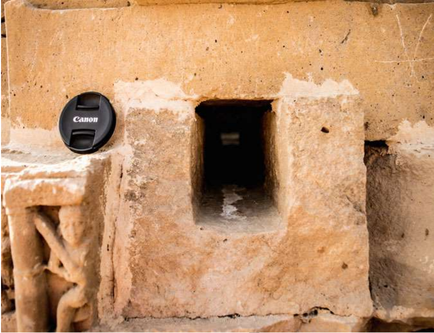
Fig. 16 Water outlet along north–south direction of width 8.1 cm and length 20 cm (Temple no. 1) (Canon cap marker of diameter 5.4 cm)
