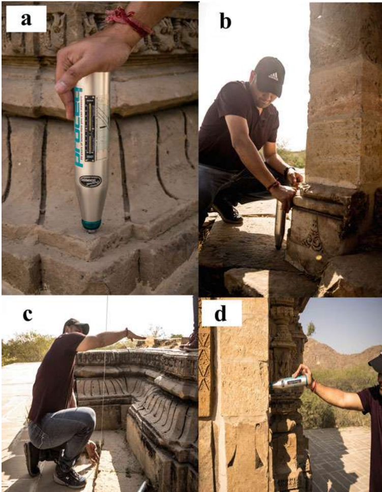
Fig. 28 Strength measurement with Smith Hammer at the Shiva Temple (Temple no. 4) for a first foundation stone, b base of the pillar, c Height (from the base of the pillar to the section where the smith hammer is kept) and strength measurement at the base of the Garbhagriha (From Bhitta to Grasapattika), and d strength measurement at the pillar
